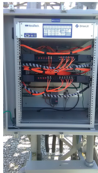
Panel in the substation yard with modern fiber optic cabling to the IEDs
