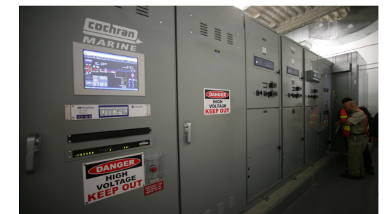
Cochran Marine Shore Power Switchgear
